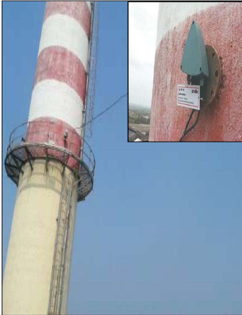
Online Monitoring System
